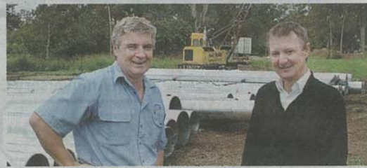
Danny Lynch from Bellerio Constructions (left) and developer Ron Blyth oversee the delivery of steel pylons, the first materials to arrive on site for a $30 million marina on the Mary River.
